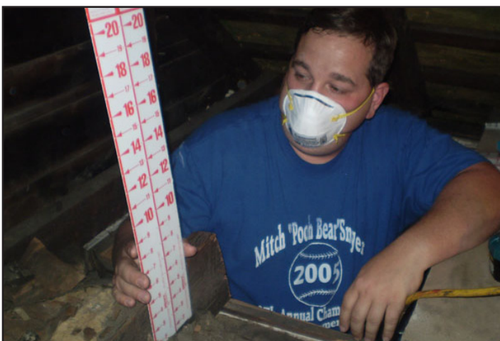
Ray Feikert, HWAP Supervisor with Kno-Ho-Co Ashland Community Action, holds a flag which will measure the 18 inches of insulation that will be blown into Ms. Smith's attic.
