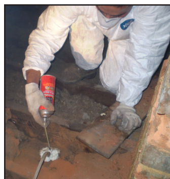
Garrett Feaster, in training for LEADS, seals a crack in the attic. Cracks like this were sealed from the attic down to the basement to stop infiltration and seal Ms. Smith's home.
