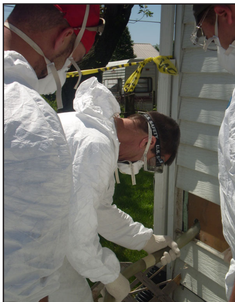
COAD Trainer Joe Ryan demonstrates technique for blowing insulation into an exterior wall. Hands on experience working at a client's home is an essential part of the Basic Weatherization Tactics class.
